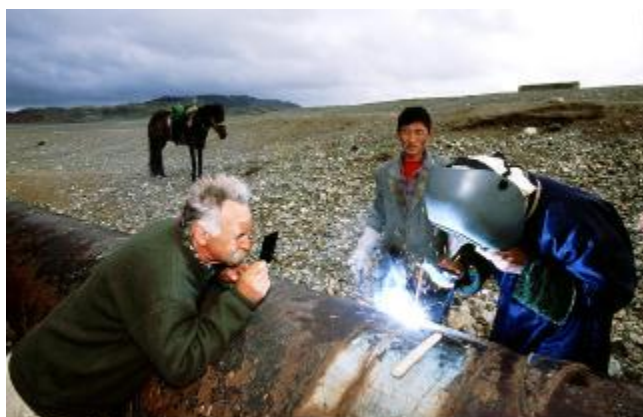
Fig. 11: Sepp Gölls supervising the repair of the defunct Russian water pipeline in Takhin Tal.
